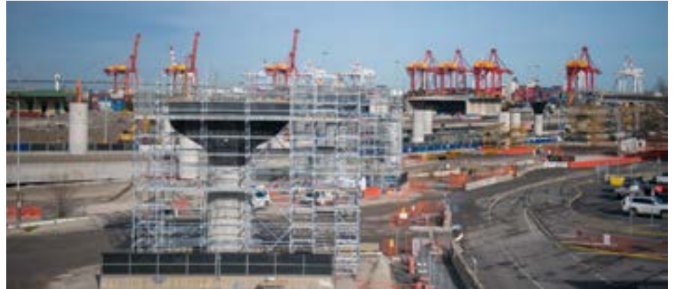
▲ Columns for a new exit ramp have been taking shape as work gets underway for an elevated roadway over Footscray Rd.
