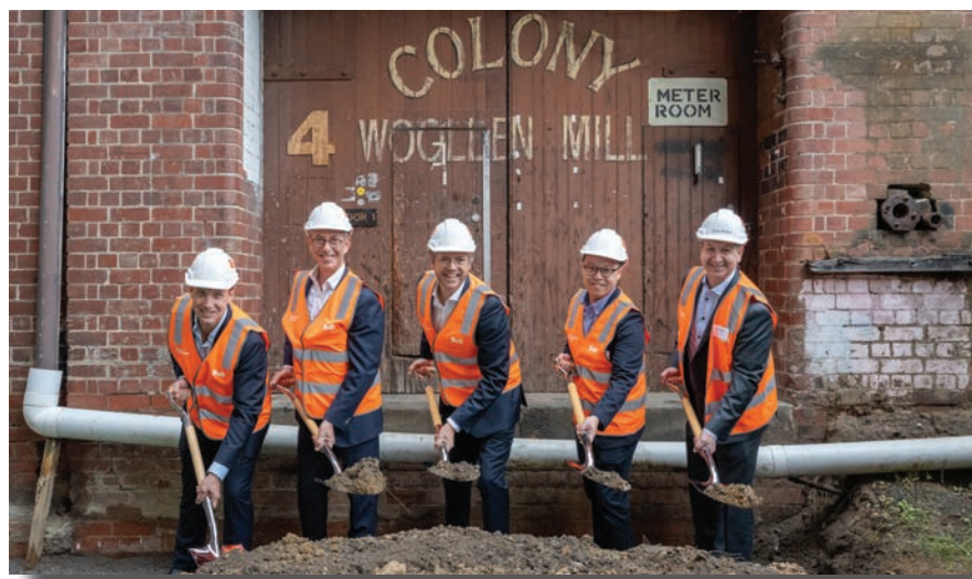
▲ April: Construction gets under way on the redevelopment of the historic Younghusband site in Kensington.
